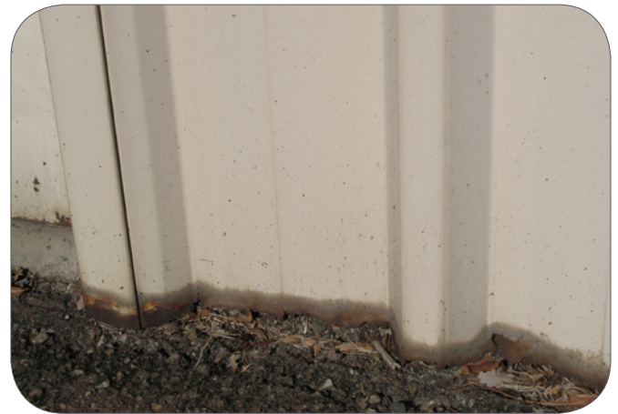
Figure 2: Corrosion due to inappropriate wall design
